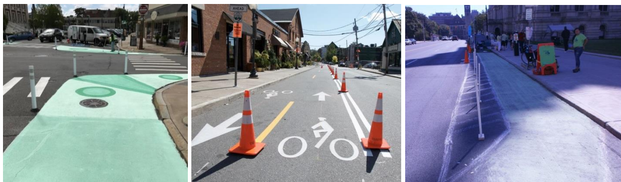
Left: An intersection enhancement project at Jay and Liberty Streets in Schenectady; Middle: Henry Street Bike Lane Demonstration in Saratoga Springs; Right: Protected bike lane demonstration at Parking Day in Albany
