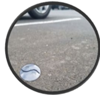
Figure 3 Smart sensor installed in street pavement
